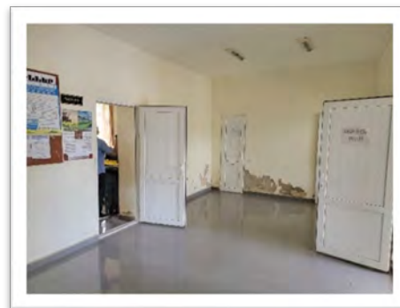
Lobby Area (in need of repair)
